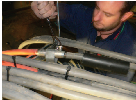
Tim Kennedy of Aotea Electric - finding low voltage cable jointing in confined spaces much simpler when using the Nexans GPH shear bolts connectors.
