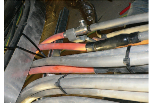
Typical example of cable installation in confined spaces under low voltage switchboard rooms.
