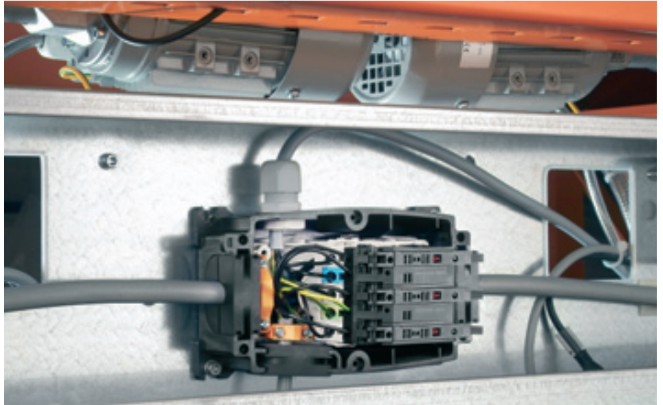
FieldPower's PowerBox integrates power supply, extension, outgoing motor feeder and distribution in a single module and can be mounted anywhere handy to the device being powered
