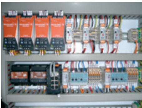
CSL offers a full range of Weidmuller modular power supply, Ethernet and connectivity solutions as seen in this Solid Energy panel
