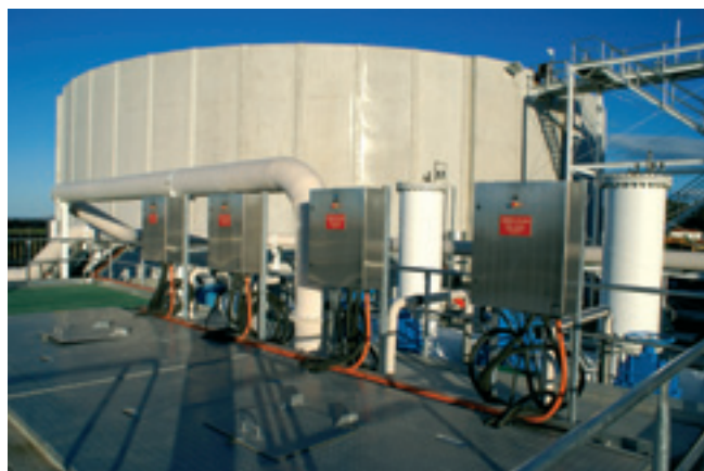
An innovative new water treatment process combined with time pressure to complete the project meant CSL and Stewarts Electrical Supplies had to make sure their recommendations performed faultlessly from the outset
