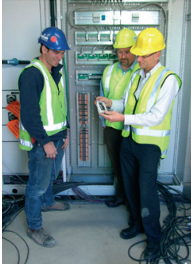
CSL's Geoff Thomson (right) provided technical advice on signal isolation for Andrew Stiver of Stewarts Electrical Supplies and Brad Jarvis of Falcon Electrical. This led to Weidmuller WavePak and ITXPlus signal isolators being installed throughout the Clive waste water treatment plant
